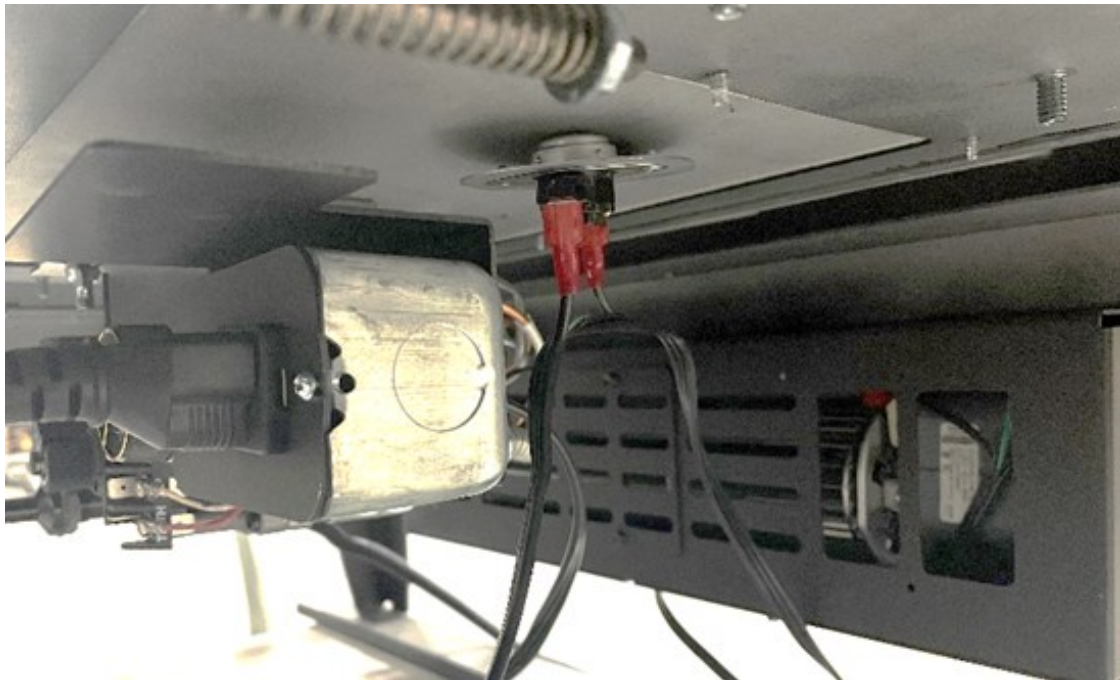
Figure 7.9, Temperature Control Switch Location
